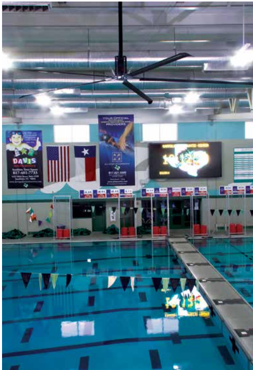
Industrial fan as used in a large aquatic center.
