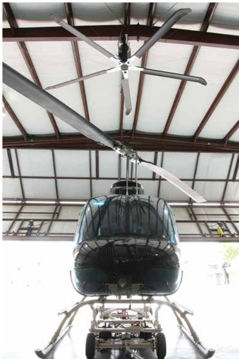
HVLS fan used in industrial hangar to provide air movement for comfort and keep surfaces dry for safety.
