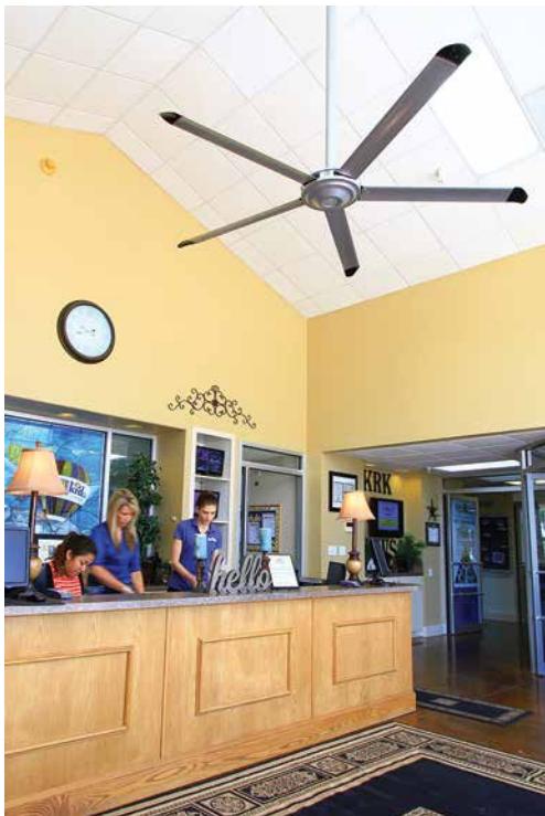
Commercial HVLS fan used in reception area of daycare facility, which helps push air down from high ceiling.
