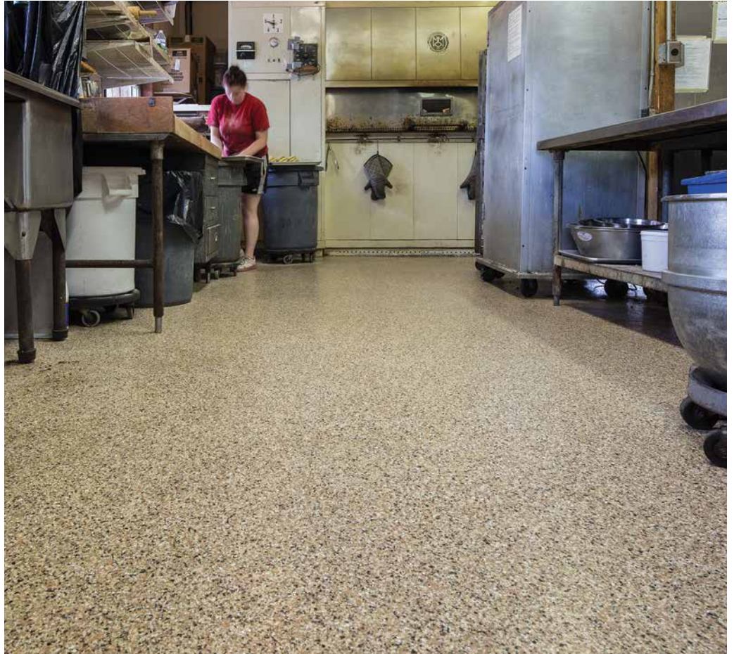
The end result is a seamless floor with a visually appealing finish that can handle the daily demands of a commercial bakery.
